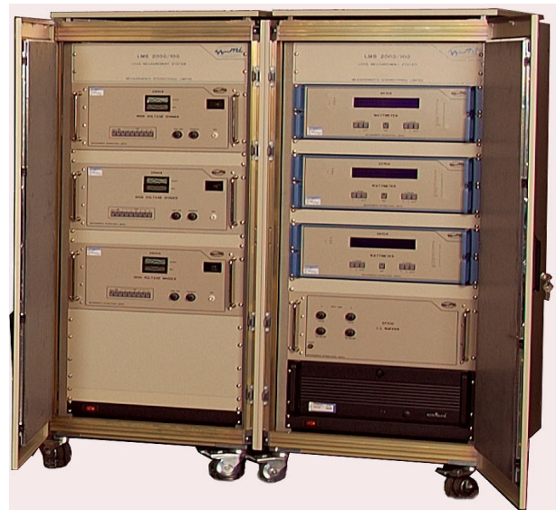
(Control Cabinet with Components)
